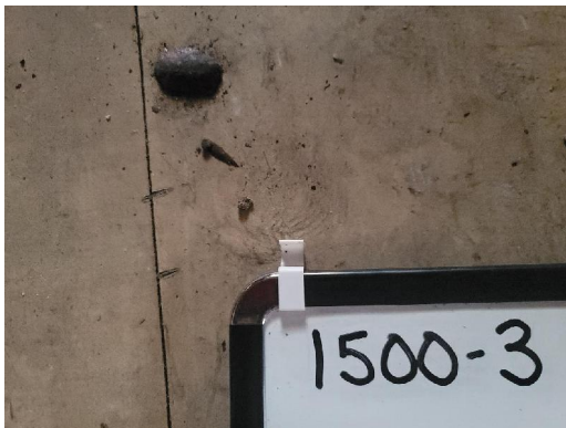
1500-3 12"x12" Floor Tile/Tan (2% Chrysotile) Mastic/Black (4% Chrysotile) Typical Interior (Bottom Layer) Appx. 650 sf
